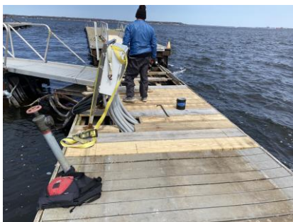
Installing 2x12's as a temporary dock surface until the repairs are completed on the steel structure of the fixed dock
