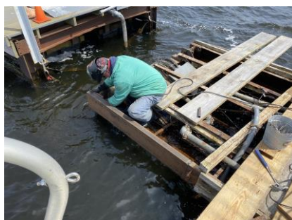
Tim Wallace repairing the east end of the fixed dock steel structure by repairing the broken welds and weldina
